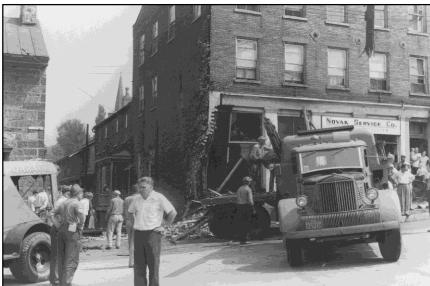
W. C. (Red) Giles stands with hands on hips as workers clear wreckage from the Shupe building.
